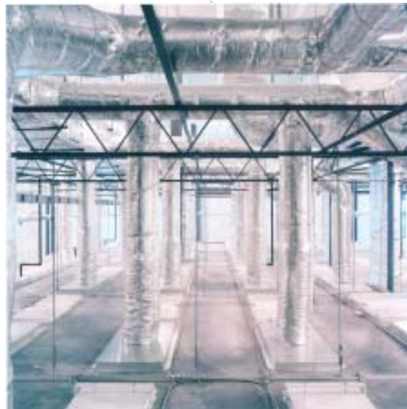
Typical Walk-On Ceiling
